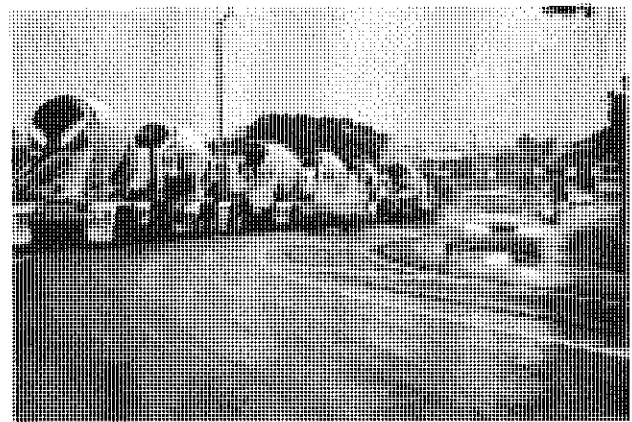
CONCRETE FORMS SET UP ALONG TAKAKI DRIVE PRIOR TO THE START OF A MAJOR CONCRETE POUR ON PROJECT HOBSON'S GRAPE CRAWL SITE. APPROXIMATELY 100 TONS OF REINFORCING BARS WERE SET UP IN A SINGLE POUR TO FORM THE BASE SLAB OF THE NEW PUMP STATION
