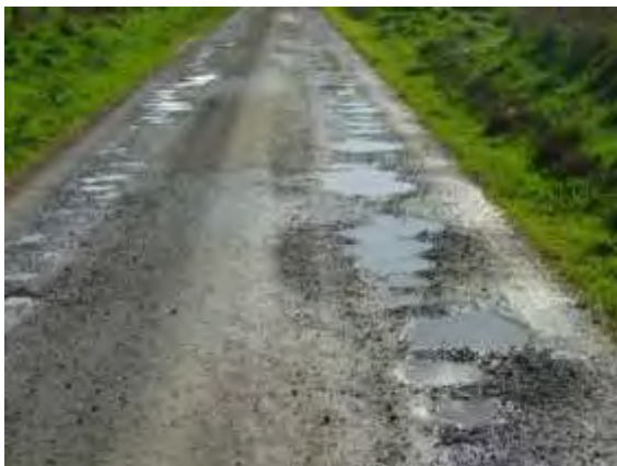
Unsealed Road prior to Resheeting
